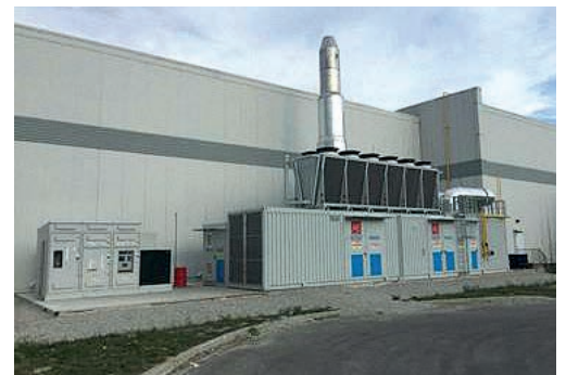
3.3 MW EPS AB Energy Canada's "GA Buster", currently operating 5-10 hours during projected peak days to ensure GA avoidance and cost savings
